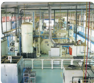
Heat Treatment Plant
